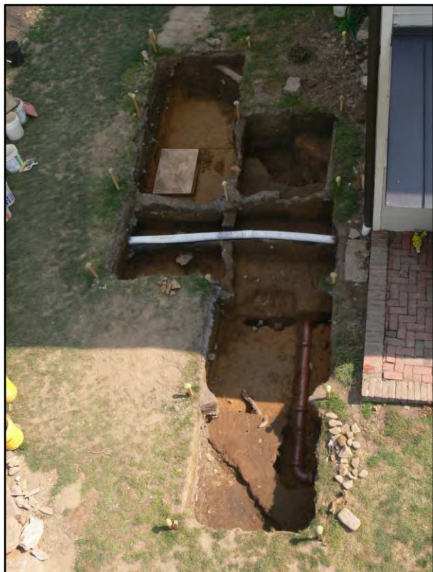
Overhead view of excavations near the brick porch at the northwest corner of the mansion house, illustrating the modern sewer pipes
