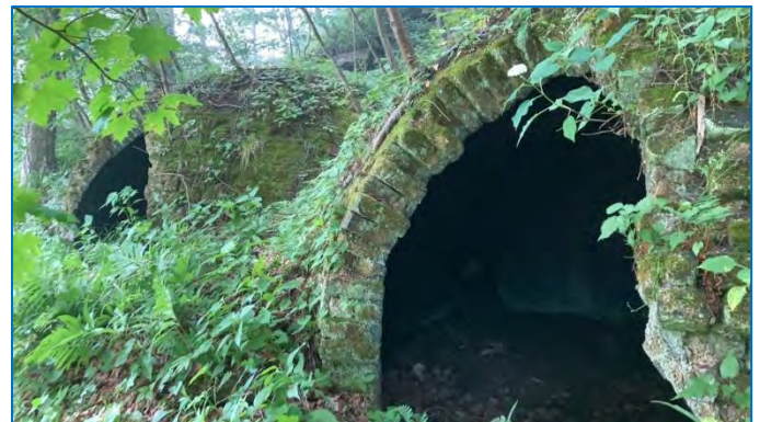
Kelly Station Coke Ovens (36AR0601) in Armstrong County. Recorded as a result of baseline survey in 2022.
