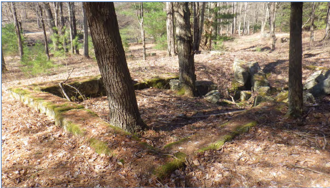
Figure 16. Cut stone foundation known as Locus 2 looking north, Clarion River in back at site (36Je200).
