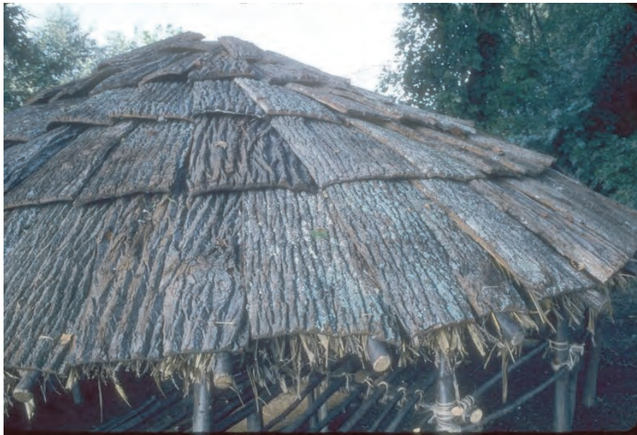
Figure 6. Exterior view of conical roof covering of cornstalk liner and bark shingles.
